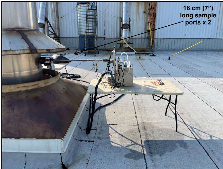
Figure B4: T105 Forehearth Stack (Source B38)
