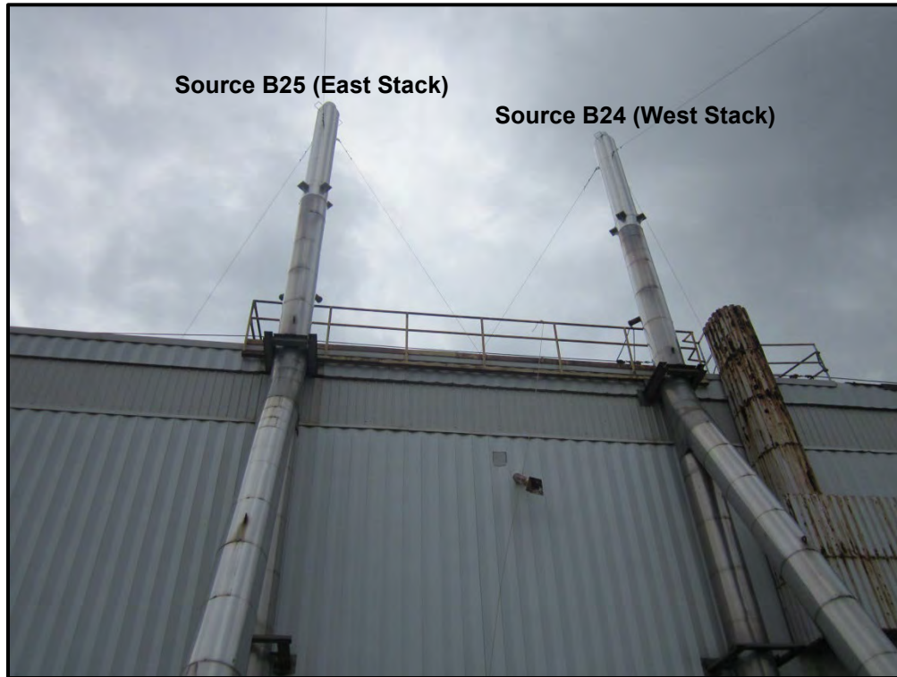
Figure B1: T105 Furnace Stacks (Sources B24 and B25)
