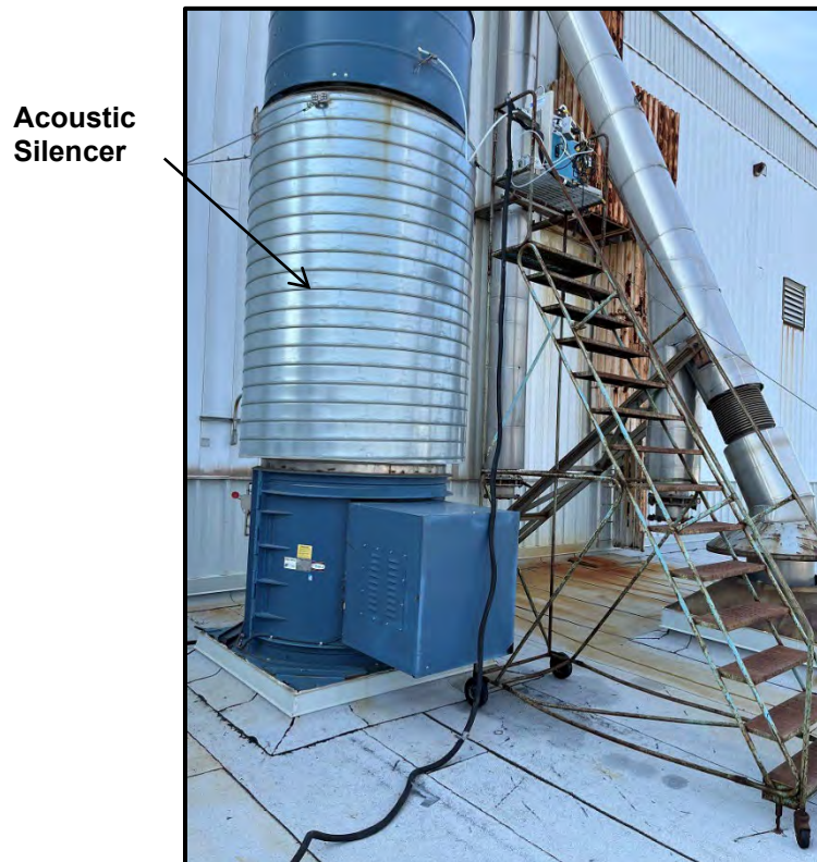
Figure B6: Furnace Hall Ventilator Style 2 (Sources B33 / B34)
